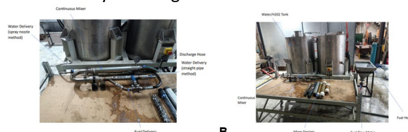
A. B. Figure 2. A & B. Elquip's rapid modification prototype test mixer platform completed. This unit has temporarily utilised the framework from the C27024 prototype mixer, and reused components of the C25005 mixer. [Image acknowledgement: Otto Lambe, Elquip]
